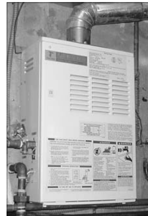
This is the tankless hot water heater installed at the CBG.
