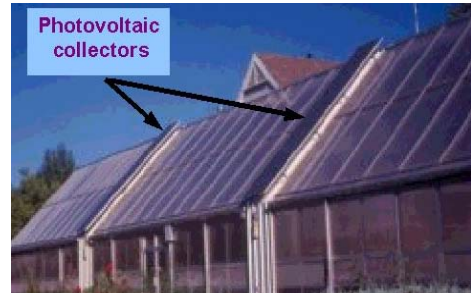
Solar electric collectors (the solar arrays) on the CBG conservatory
